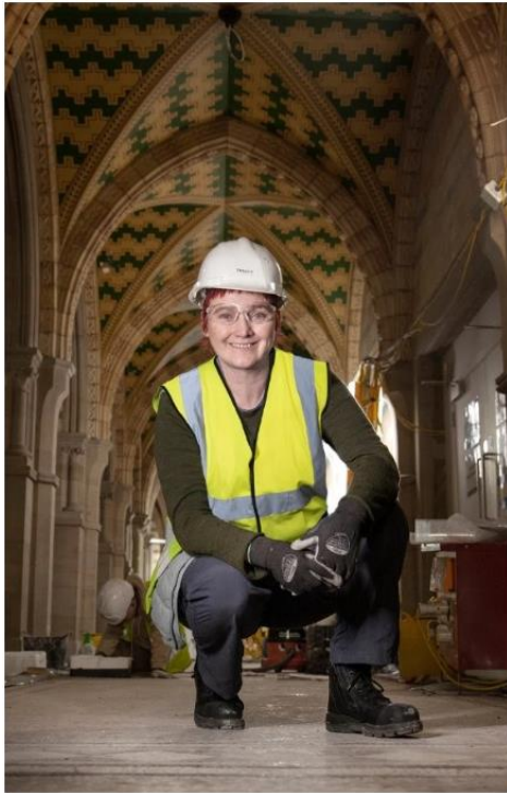
Tracey Cartledge, of Mosaic Restoration Company, working on the Manchester Our Town Hall restoration.
