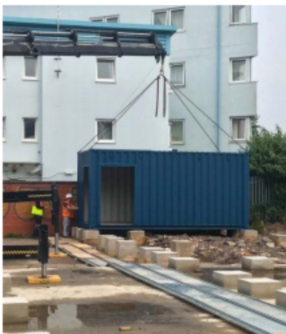
Shipping containers used for emergency accommodation
